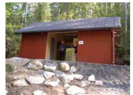
The new toilet at Haukkalampi, in the Nuuskio National Park was built on site.
