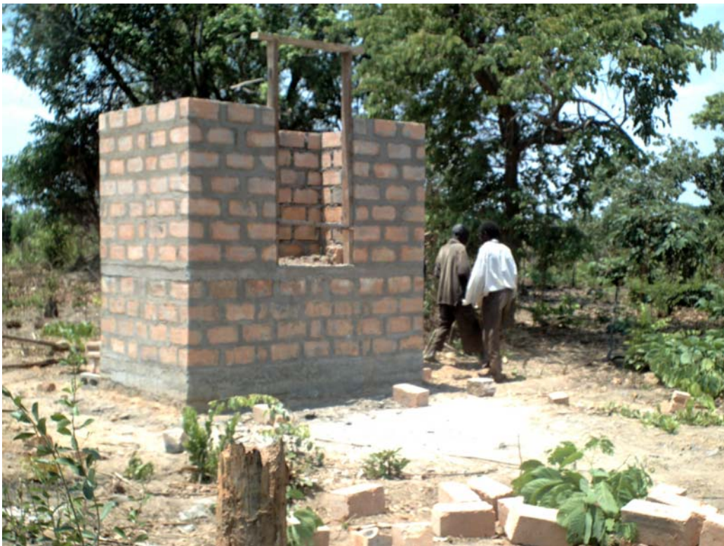
Running away from community work? An incomplete Dry toilet at Kasamwa
